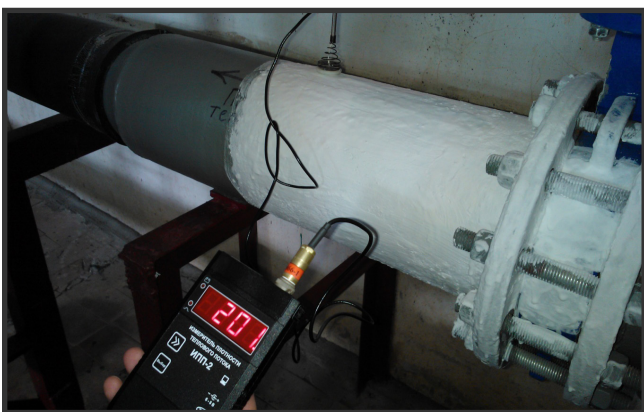
Hot - Cold Pipes
